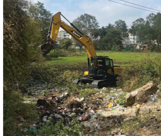
Above: The lake rejuvenation process began with the removal of waste and sludge using heavy machinery.
